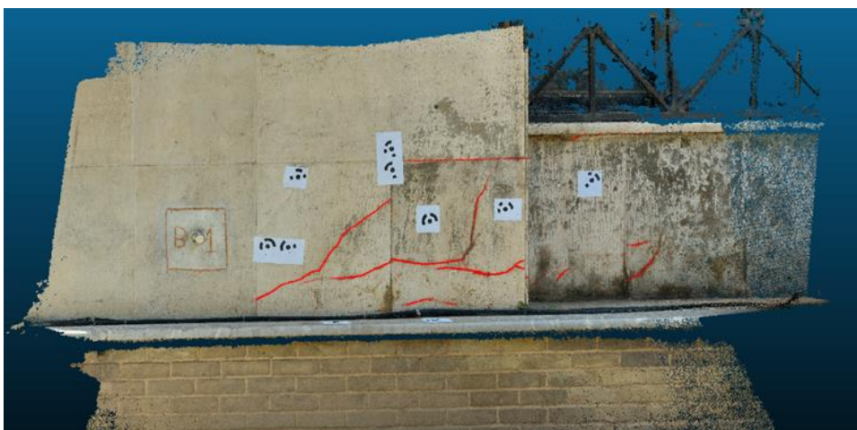
3D DENSE POINT CLOUDS AND DEPICTION OF 3D RECONSTRUCED CRACKS WITH RED COLOUR.
